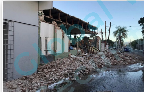
Structural damages (Washington Post, 2020)
