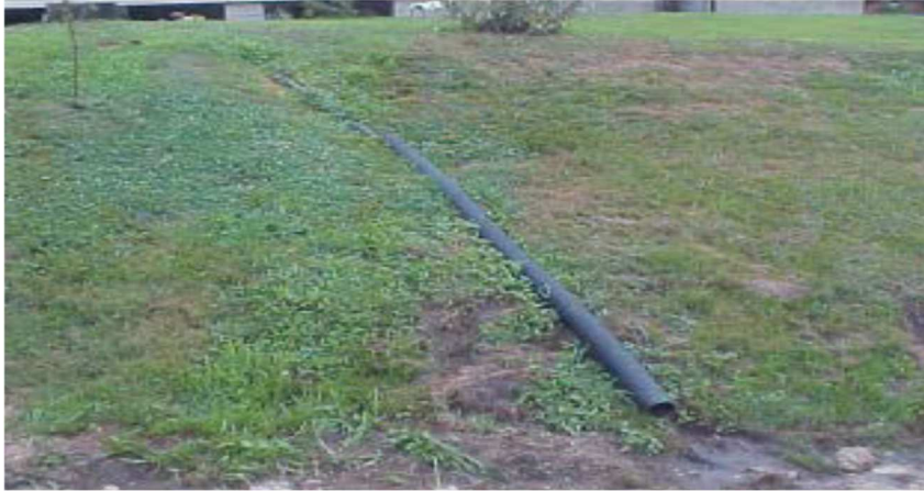
Figure 2. A Typical Straight Pipe Discharge (EPA Region 4, 2002).
