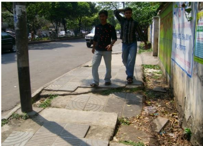
Fig 3.1: Poor condition of footpaths of Dhaka City
