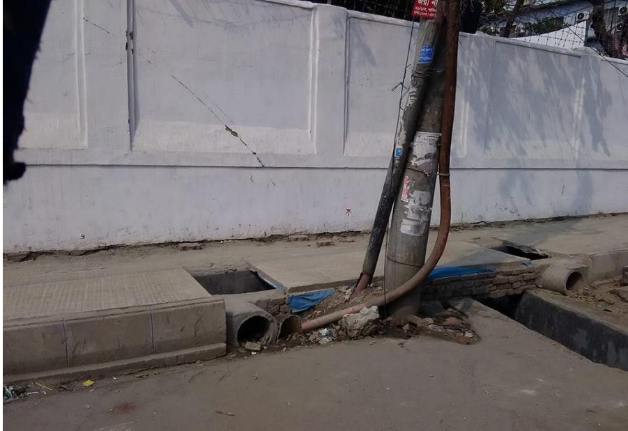
Fig 3.2: Poor condition of footpaths of Dhaka City
